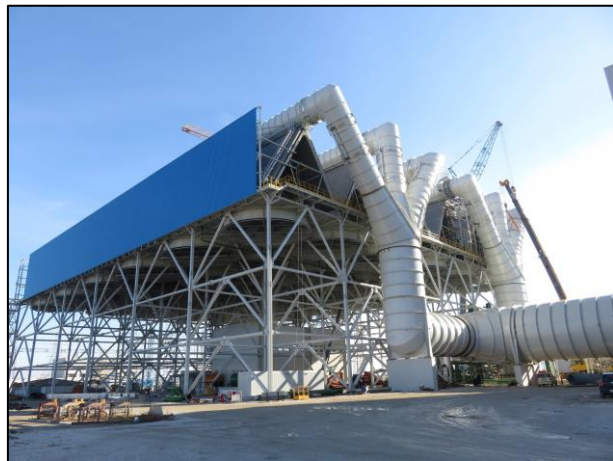
Air-Cooled Steam Condensers
